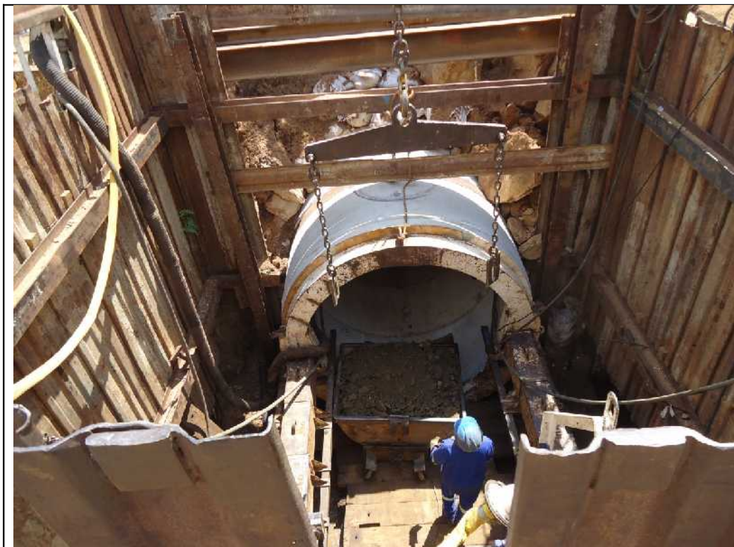
Outlet tunnel is constructed by means of pipe-jacking to overcome expected weathered zones.
