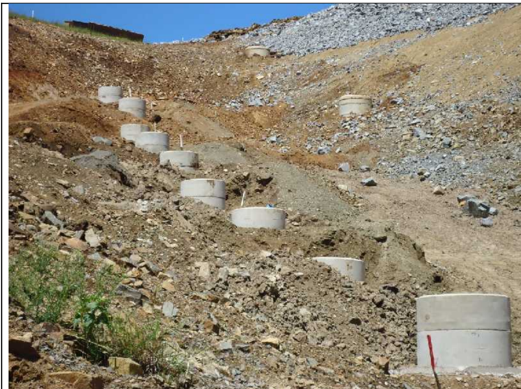
Picture shows line of pressure relief wells on LHS and conventional toe drain on RHS, at downstream embankment toe.
